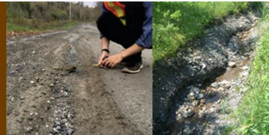
Erosion problems on roadways in the Lake Memphremagog watershed
