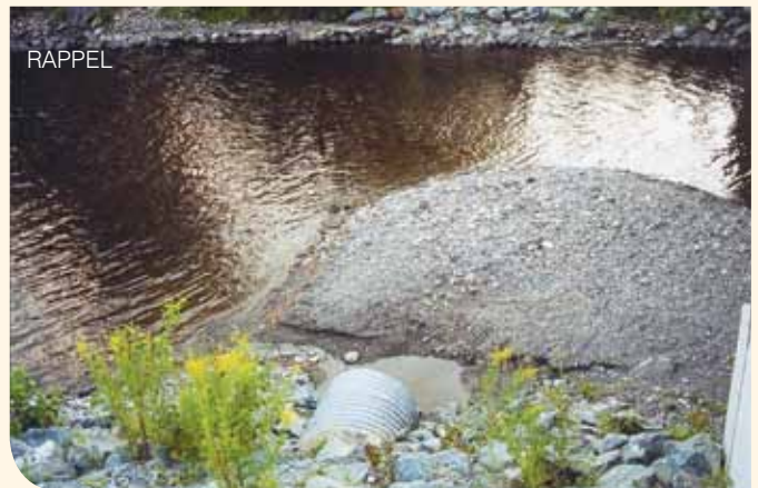
Spawning bed buried under sediment from an eroded ditch, Route 222
